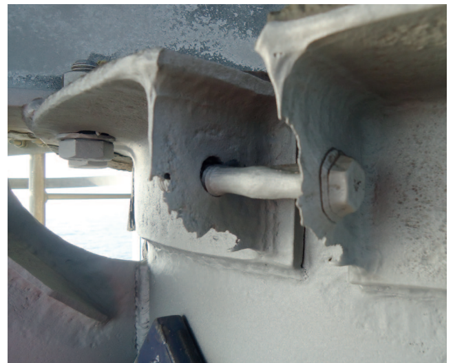
Detail of extent of corrosion to steelwork below main walkway section after blasting works completed.
