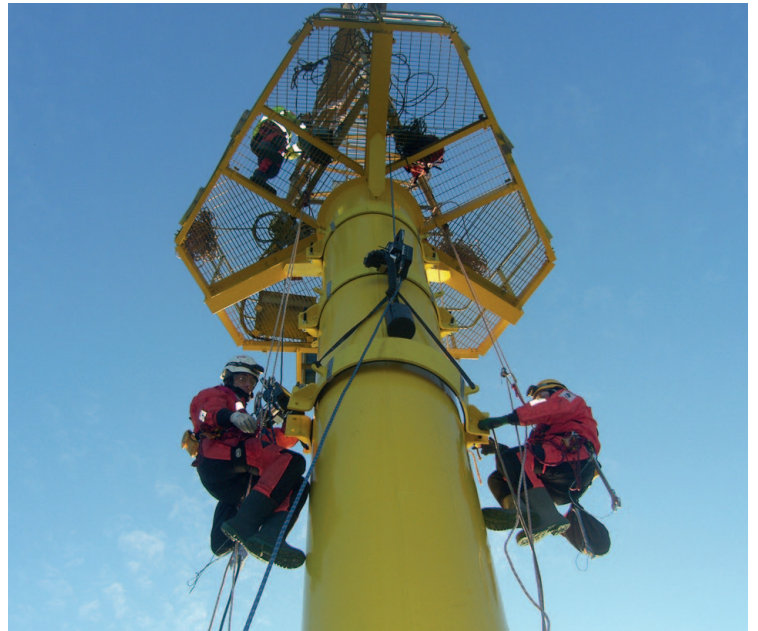
Newly fabricated Clamp sections being installed by Abfad personnel using rope access techniques.
