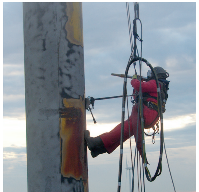
Blast operations to Met Mast stem using rope access techniques and Abfad's patented magnet system used to hold the operative in position during blasting.
