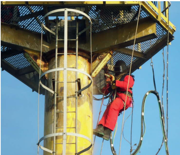
Blasting corrosion on underside of walkway and top section of Met Mast structure using rope access techniques.
