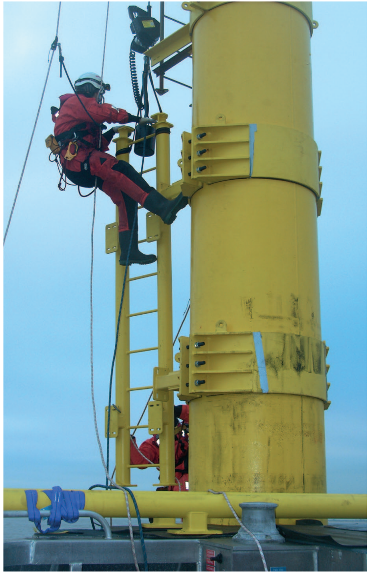
Installation of new ladder section, Abfad electric battery winch used to move and hold ladder section in place during installation.
