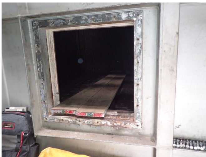
Access hatchway with scaffold boards in place to ease entry over the studs and form part of the emergency arrangements.
